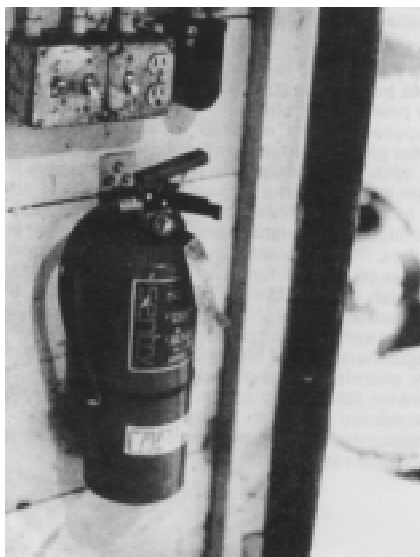
Figure 12-112 Fire extinguisher label
