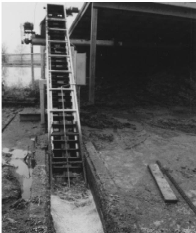
Drag conveyor loaded
