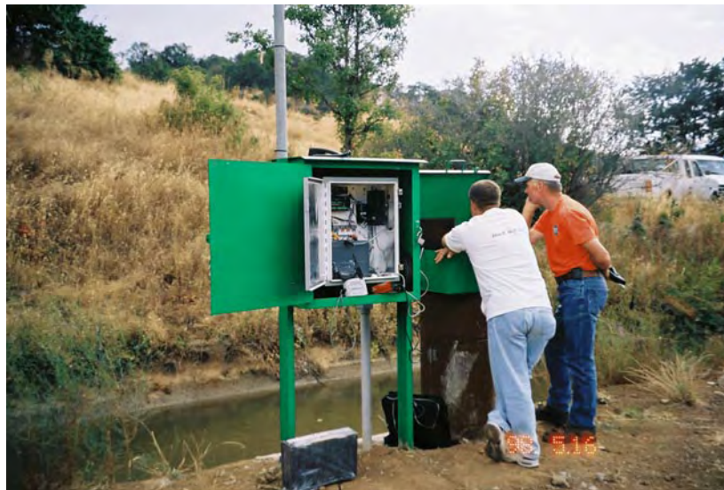
Photograph 4. This view of the site on Talent Canal shows the equipment cabinet containing the data logger and dial-up equipment. The technicians are installing the float well equipment which was used to verify the depths obtained from the pressure transducer in the Starflow instrument.
