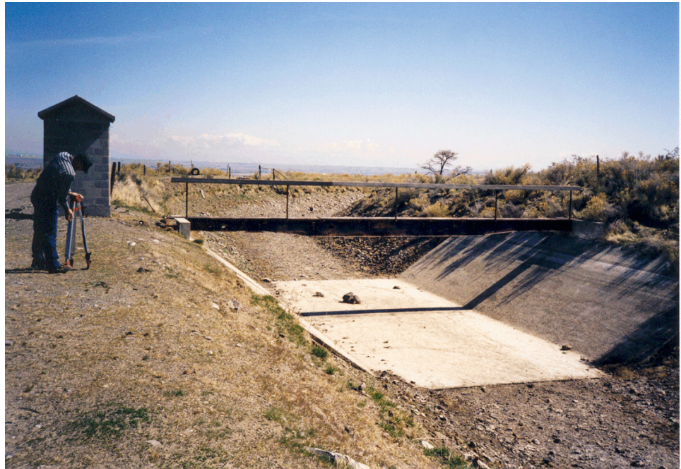
Photograph 5. The view is looking downstream at the South Canal measurement site. The StarFlow instrument was installed in the concrete section. Canal capacity is approximately 500 cfs. This site was chosen because there is a well-defined, stage-discharge curve which could be compared with the data gathered from the demonstration instrument.
